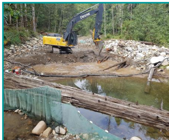
Digging out the bedload. Sediment control and fish nets in place to protect the water quality and stop fish from entering the site.
